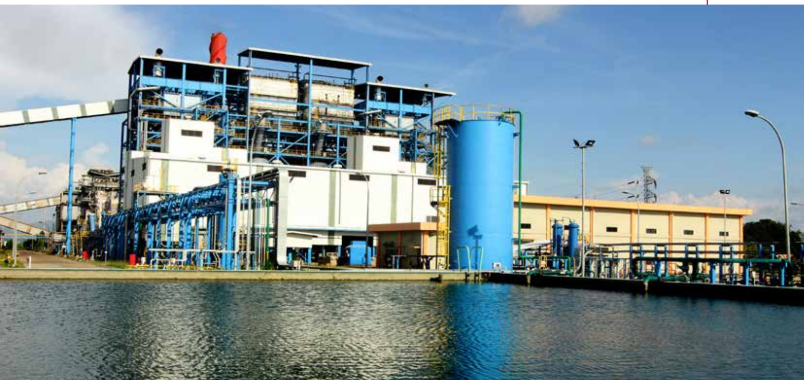
Boiler turbin generator unit 2
